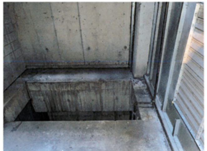
Unguarded shaft opening which employee fell into.
